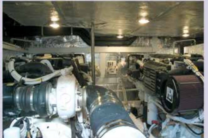
CLOCKWISE Crew Cabin. Detail. Engine Room.
